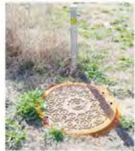
Manhole cover marking
