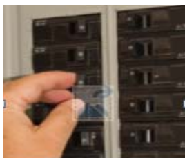
Locate the correct energy isolation device
