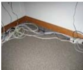
Never connect extension cords/power strips to each other.
