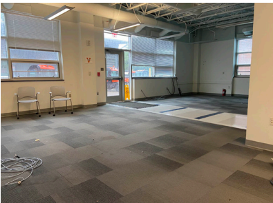
The start of the Skipwith Hall lower level renovation, June 2023. Photo provided by Emily Douglas.
