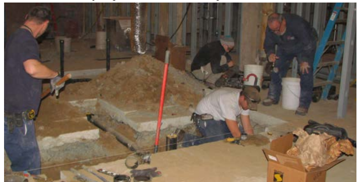
Project Services plumbers and electricians install water and utility lines in the cement floor. Working here are (L-R) Plumber Chris Morris, Plumber Apprentices Mariah Kurpel and Shane Black, Plumber Paul Johnson, and (out of view) Plumber Apprentice Dakota Peregoy.
