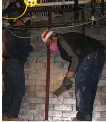
Project Services Glenn Tolbert and Matt Proffitt remove lead bricks from the old X-Ray department.
