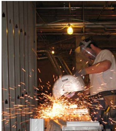
Project Services Carpentry team member Ben Collier cuts metal studs to fit the frame out for new offices.
