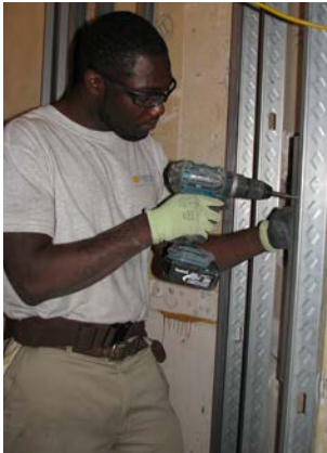
Project Services Carpentry team member Quentin Walker drills metal studs together for the installation of the drywall.
