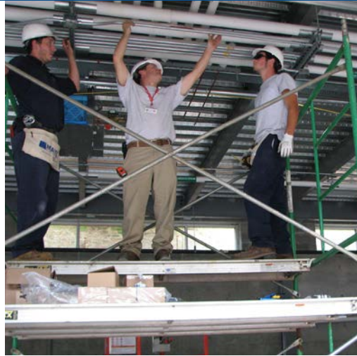
Project Services' Electrician Rob Chaffinch (center) explains to apprentices Cody Borrelli (left) and Dillon Dean how to roll electrical conduit off the rack while keeping the pipes straight.
