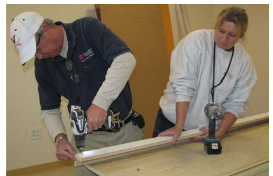
Health System Trades Carpenter Lead Blaine Derryberry and Bonnie Barnett complete an installation for the McLeod 3rd Floor renovation.
