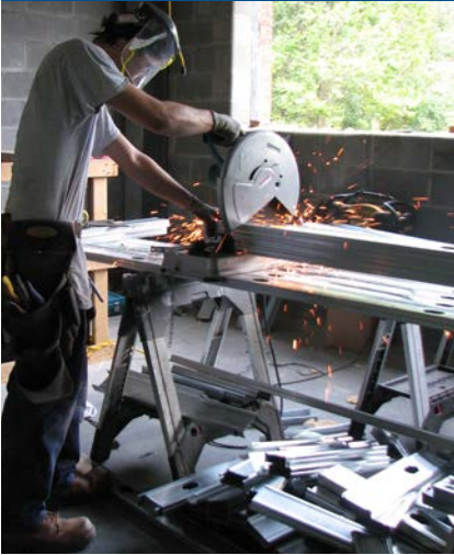
On the second floor of SEAS/FM Building (now officially named Lacy Hall), Carpentry Apprentice Matt Anderson cuts metal studs for framing. The new location for several Facilities Management shops will be occupied by early 2013.
