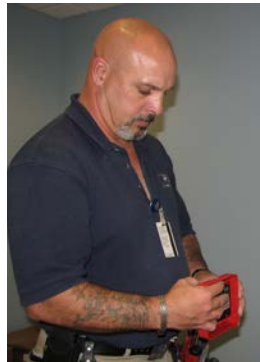
At McLeod, Fire Systems Technician Pat O'Gorman sets a fire strobe's candelas.
