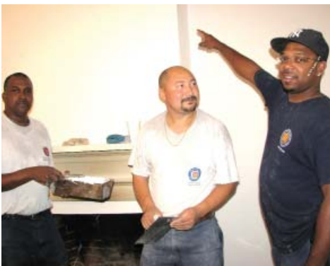
Masonry Shop members Roland Taylor, Dorjee Damdoo and Sam Amos put final touches to the walls in the Student Room by Pavilion X as
