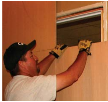
Jerry Morris sets the unstained panelling in place after occupants have left for the day.
