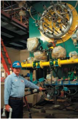
Russell DeShong shows off the first new boiler.
