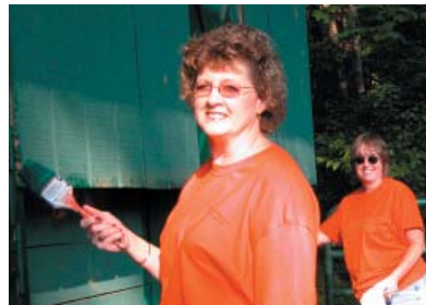
Left photo: Libba Bowling, Shaun Farrell & Bill Hodges built a deck. Above: Joyce Chewning (our United Way Coordinator) & Brenda Buttner paint stables. Right: Robert Garland, Ronnie Spencer, Lew Persinger & Brian Terrell repair walls.
