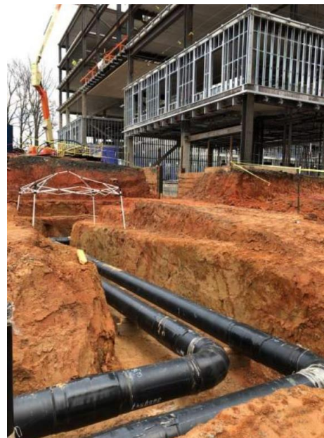
4. LTHW piping going into the UCH building
