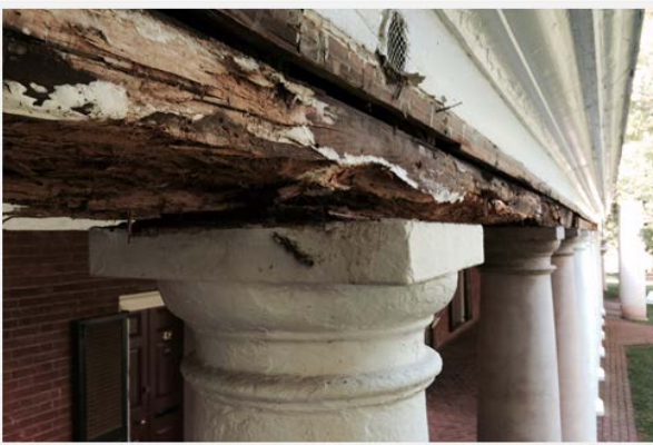
East Lawn – Recently discovered Colonnade support beam deterioration, hidden by fascia board
